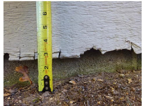
Facade finishes need to be kept a sufficient distance above grade to prevent water damage and rot
